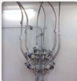
Multi-line for the feeding of the weighed cyclone; allows the production of the pre-mix during the transfer phase
